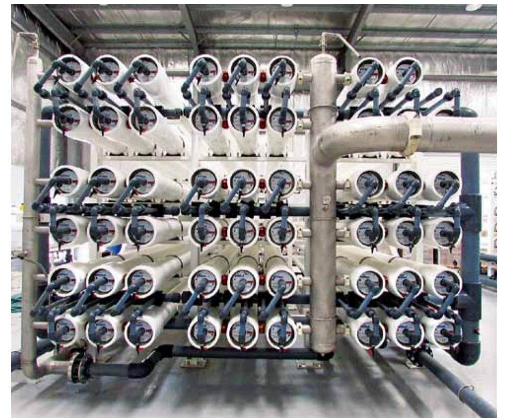
Reverse osmosis technology to produce treated water
