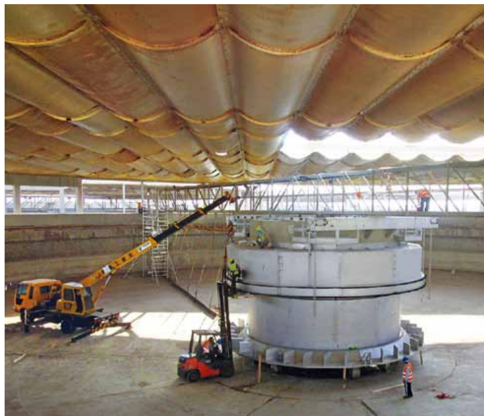
Jeddah (Airport 1) sewage treatment plant
